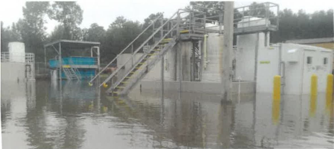
Figure 9-15 Casino Waste Water Treatment Plant
