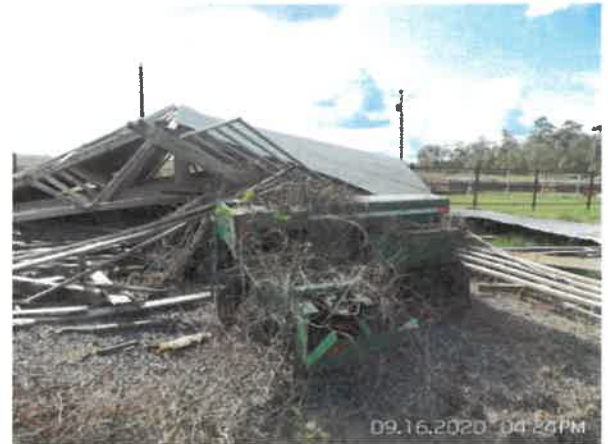
Figure 9-20 Collapsed Cattle Shed
