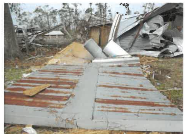
Figure 9-21 Collapsed Water Pump House
