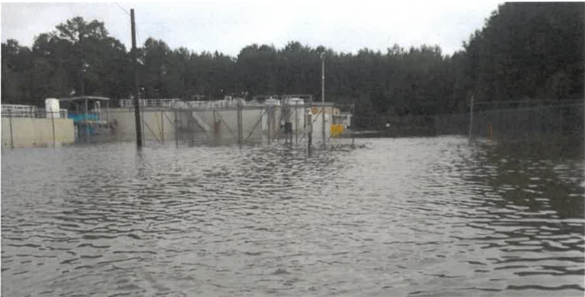
Figure 9-16 Casino Waste Water Treatment Plant
