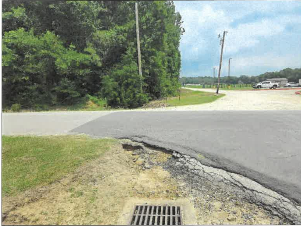
Photo 1: Road alignment center line from western tie in point to CC Bel Road facing west past Powell Road.
