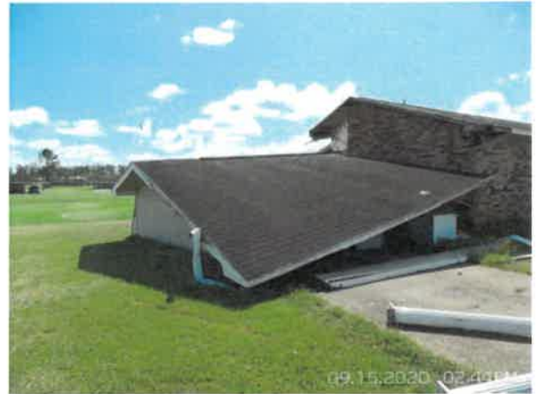
Figure 9-19 Residential Structure Roof Collapse
