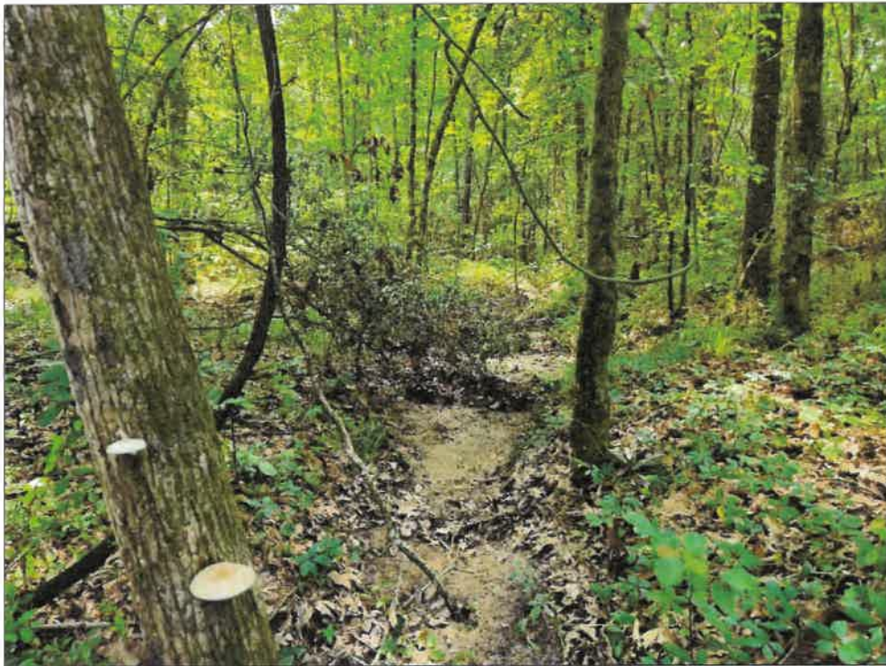
Photo 21: Downstream view of lateral drain just north of the site that discharges to Bayou Blue in background.
