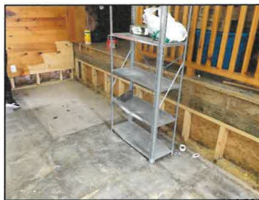
Figure 9-24 Remediation Work Required in Museum Due to Flood Waters
