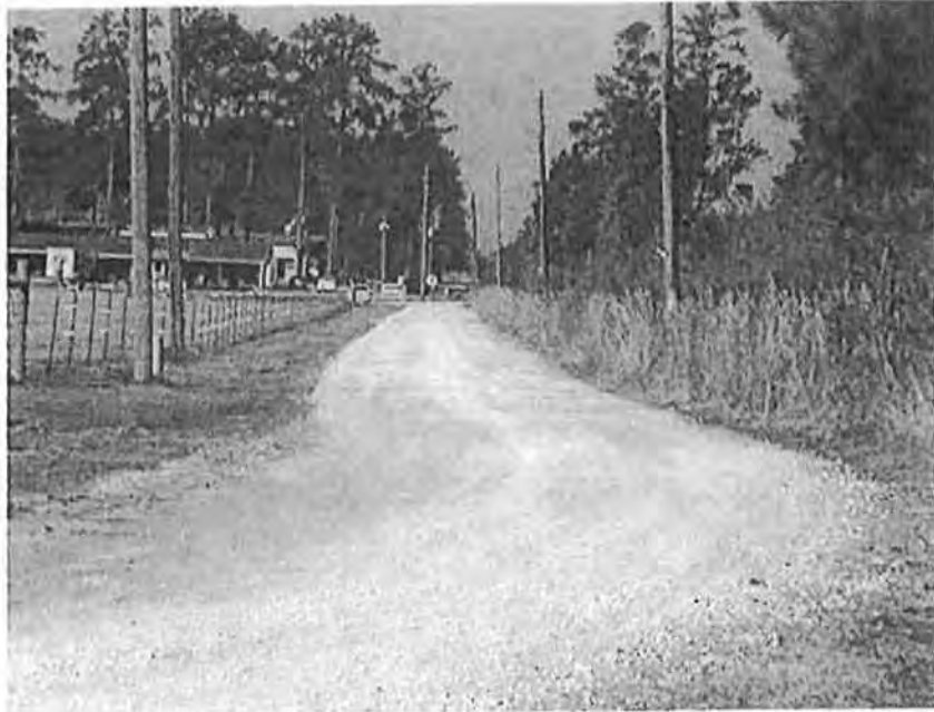
Photograph location N30°31'25.34", W92°42'36.74" (Beginning of realignment of Camp Coushatta Road Project looking toward the beginning)
